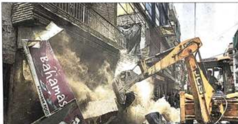
At an anti-encroachment drive in west Delhi's Shyam Nagar.
